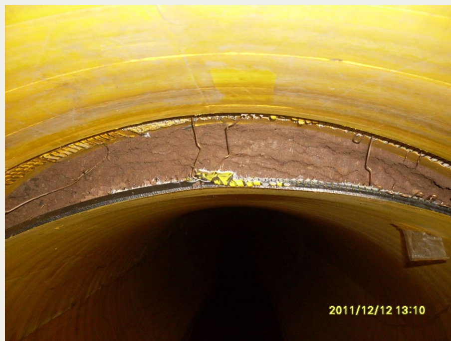
Failure – external loading
