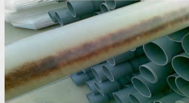
Discolouration due to degradation
