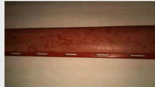
Discolouration due to "chalking" Change lubricant system, add UV resistance improve pigments
