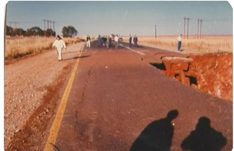
FIGURE 3: SINKHOLE ON HIGHWAY AS RESULT OF LEAKING WATER PIPE
